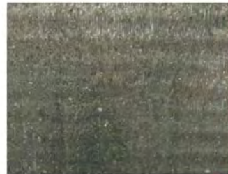
A dirty coil impedes airflow losing efficiency making the system work harder increasing energy costs
